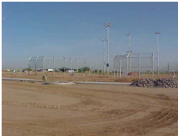
Avondale Youth Sports Complex baseball fields with backstops, fence posts and lights installed.
