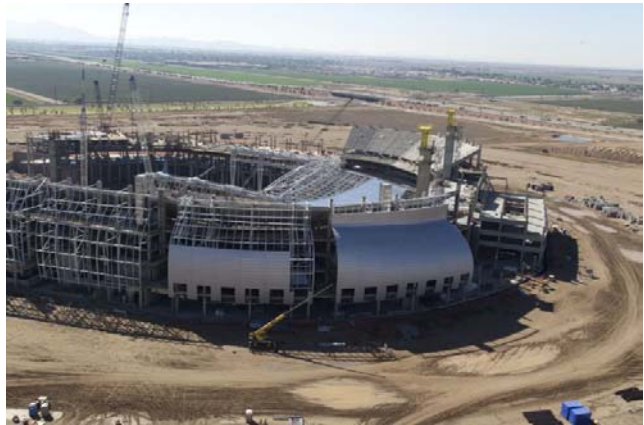
Northeast corner of Stadium showing progress on exterior metal skin and upper seating bowl.
