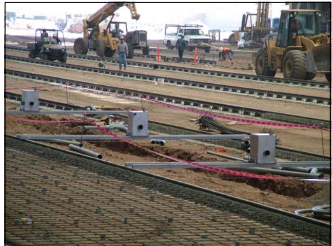
Utility grid boxes (visible in the center of the photo resting on temporary supports) are being installed under the field floor, making the stadium one of the most flexible multipurpose facilities in the U.S.
