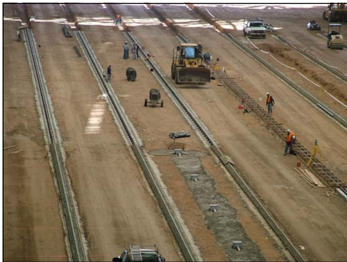
These 13 rails being completed inside the stadium will serve to support the 16.9 million pound field tray when it is rolled in for football and soccer games.
