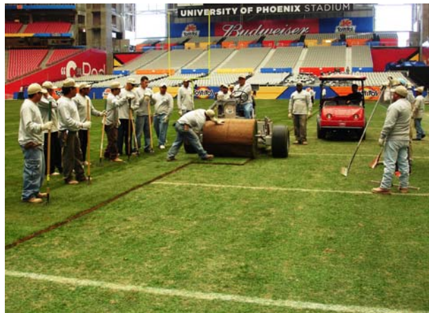
New Field Overlay — Crews install a brand new layer of turf for the BCS National Championship over the existing field used for the Tostitos Fiesta Bowl.
